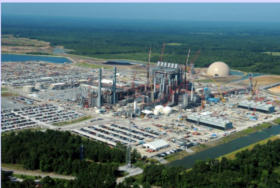
Kemper County coal IGCC power station with carbon capture, currently under construction. XTUV0010
