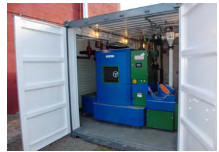
Figure 8. High-efficiency pellet boiler installed in a container outside of existing building. (Courtesy of ACT Bioenergy)
