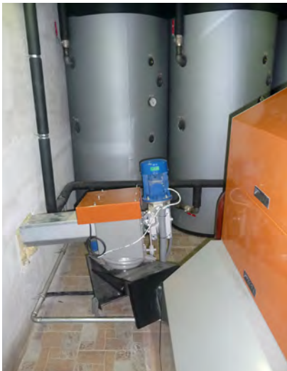
Figure 5. Thermal storage tanks and a commercial pellet boiler. (Courtesy of EvoWorld)
